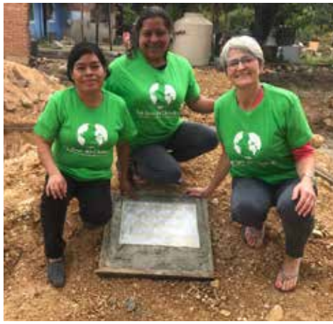
The laying of the foundation-stone – and a smiling greeting from our French and Mexican partners, wearing Don du Choeur T-shirts, who will manage the project on the ground. From left to right: Modesta Hernandez Lopez, Maria Elena Ramirez and Isabelle de Boves.
