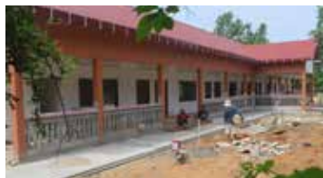
The third building nears completion; in all, 550 pupils will attend the school
